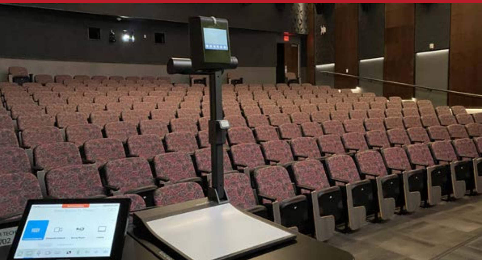
VZ-8.UHD Visualizer system installed in the campus auditorium at UNLV.
