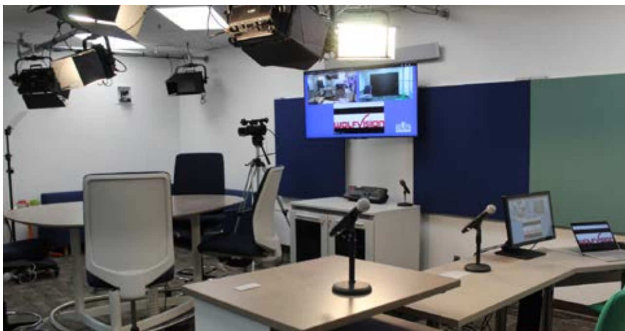
Dual wireless Shure SM58 microphones are used for audio. A Nureva HDL300 audio conferencing system is used to pick up audio from every part of the room in situations where groups of speakers are using the room.
